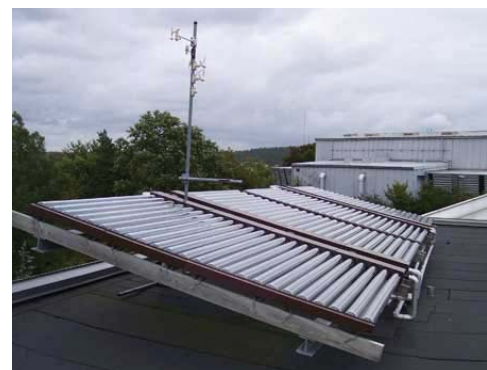
Solar water heaters
