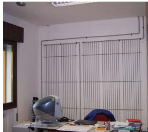
Radiant wall heating
